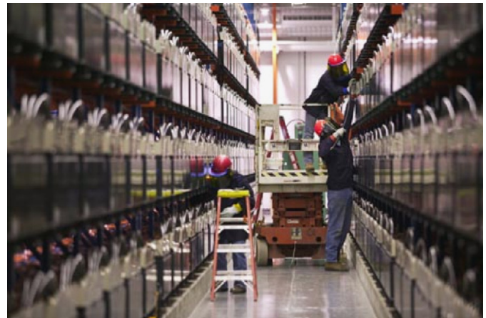
Fig. 1. The world's most powerful battery, at Golden Valley, Alaska, provides back-up to an isolated electric power system. Picture courtesy of Golden Valley Electric Association.
