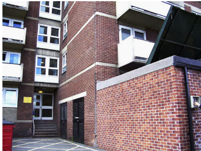
Fig. 1. Britannia House, Barnsley—new woodchip fuel store shown on right with raised delivery hatch.
